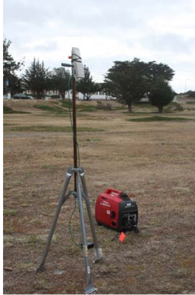
Figure 49: Wireless mesh access point, mast, and portable generator [color online]
